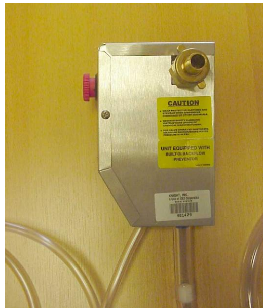
Mixing device switched on
